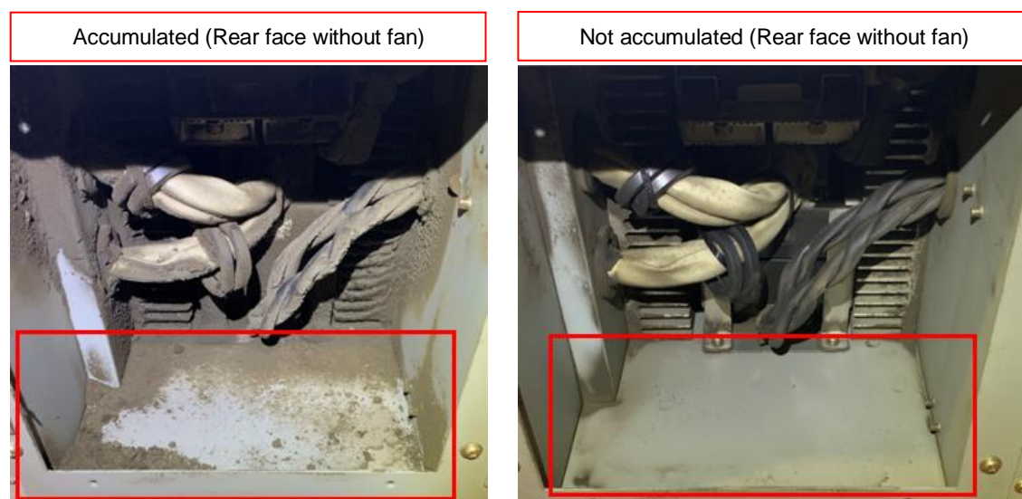
Fig. 3-3: Accumulation of Dust and Dirt (Bottom)
